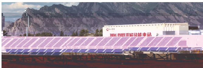
The high-performance lead-carbon battery energy storage project
